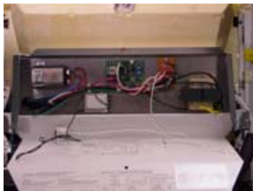
FIGURE 28. Electrical Box 1x Single Transformer
